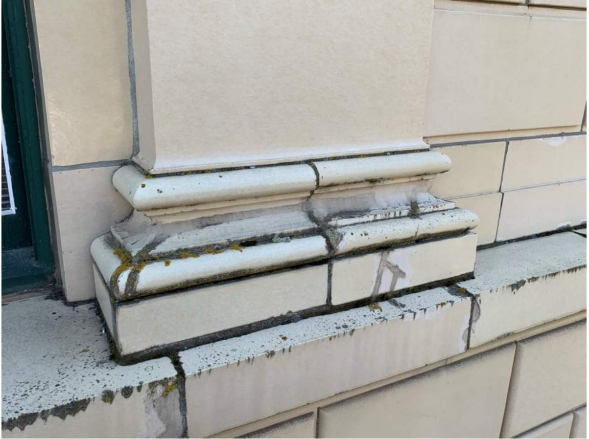
Figure 5 - Terracotta - Existing Conditions
