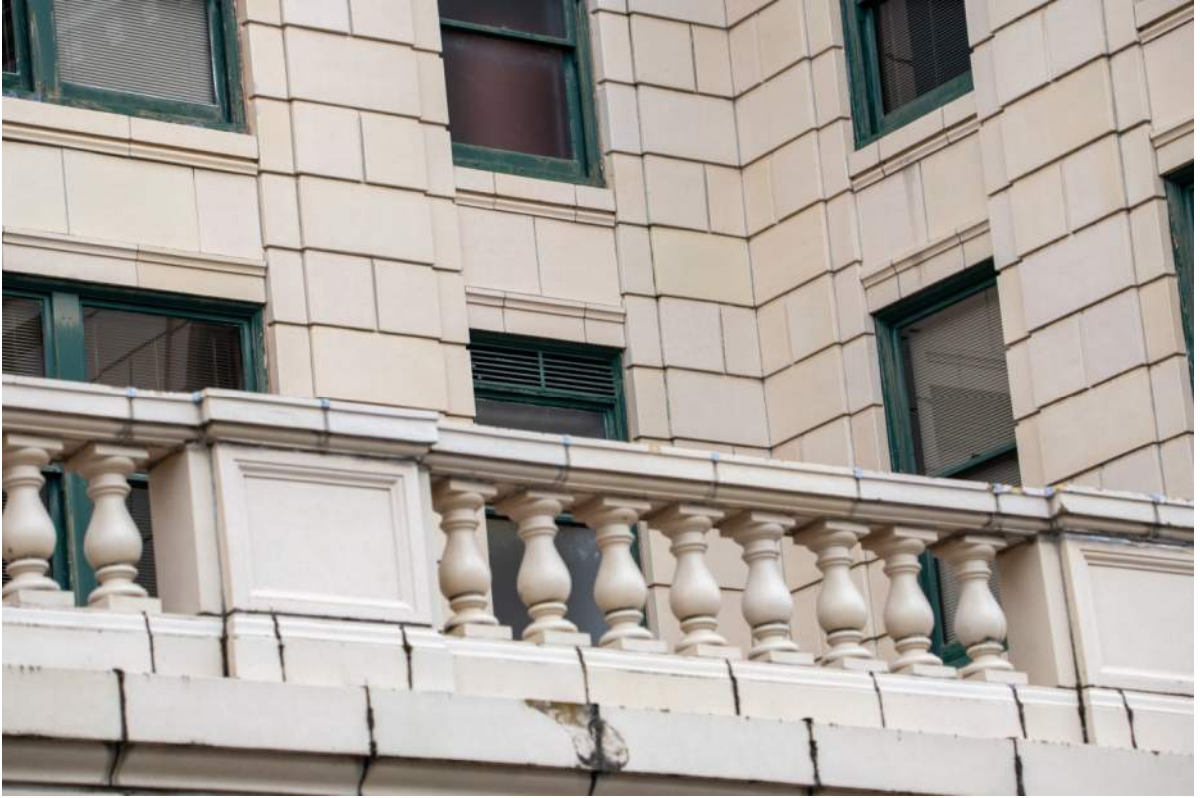
Figure 6 - Terracotta - Existing Conditions
