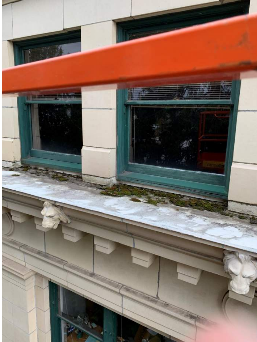
Copper sill pan flashing(painted white) below the wood sill under North façade 5 th floor window. Distance from sill pan varies from left to right as the roof slopes.
