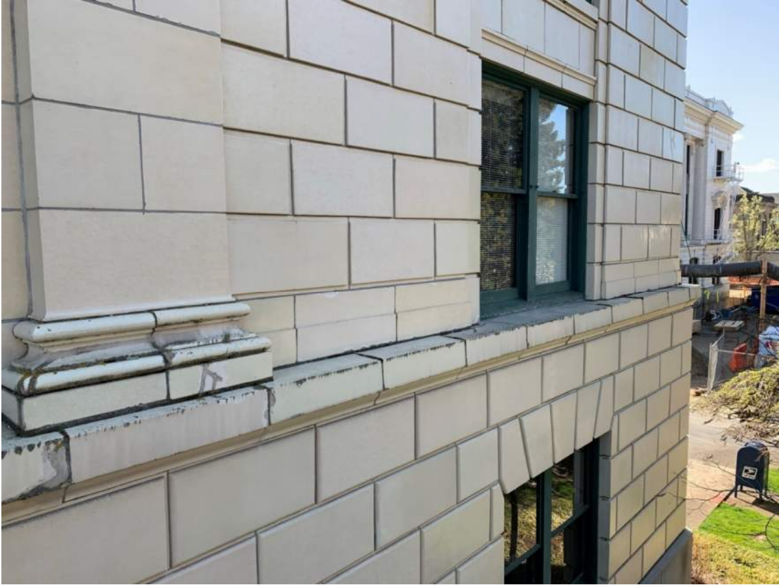
Figure 4 - Terracotta - Existing Conditions
