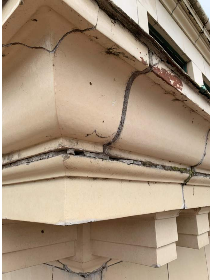
Figure 7 - Terracotta - Existing Conditions at Cornice
