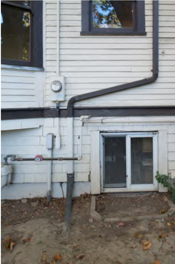
Illustration 8: Existing Electric Meter, West Side of House Off Kitchen
