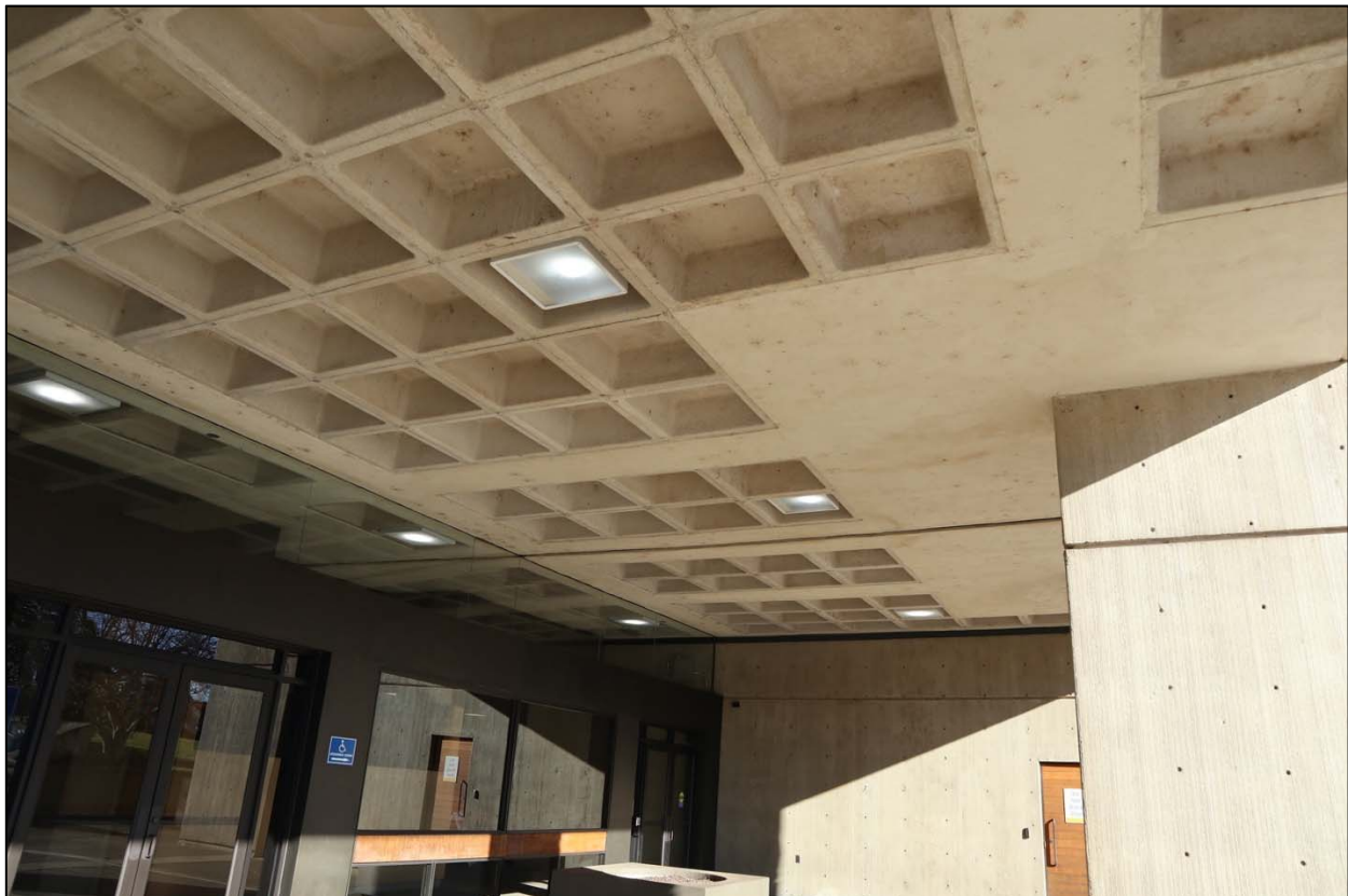
Photo 20 of 40. City Hall waffle slab construction in the front entry, looking east.
