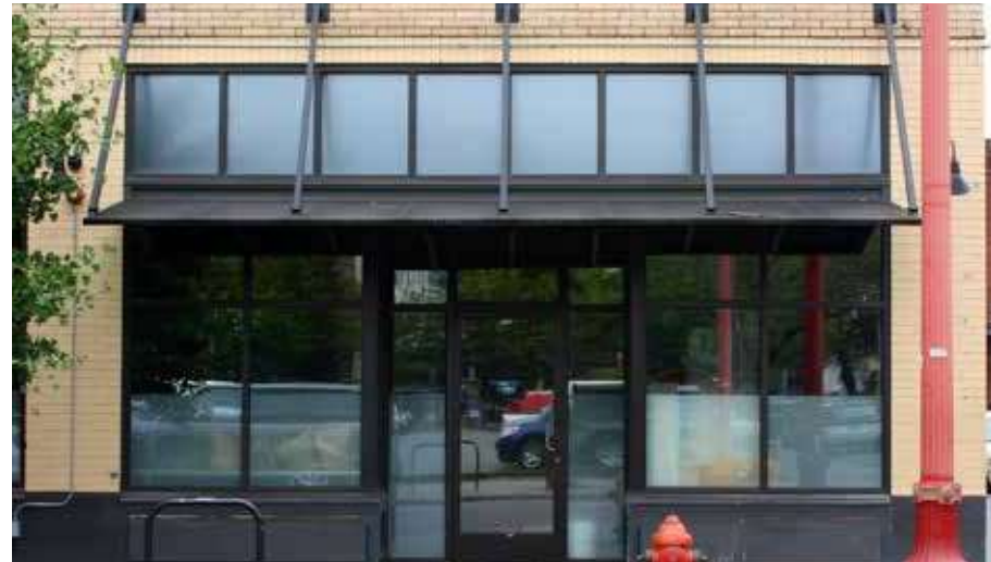
These projecting awnings at Block 28 allow the transom windows to remain visible.
