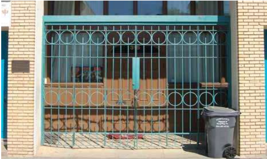
The folding security gate at the Chinese Consolidated Benevolent Association was designed to fit its opening with minimal impact to the storefront and adds Chinese decorative detail to the entry.
