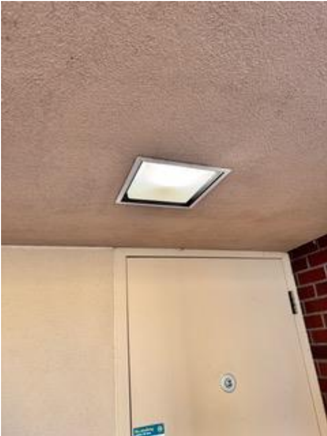
Visualization of installed lighting
