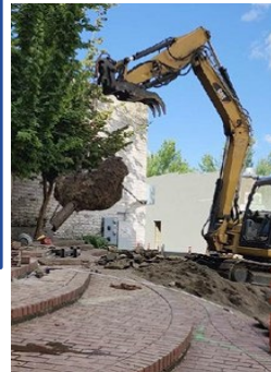
Excavating to reach the broken line at City Hall, Peace Plaza side. (Photo at right).
