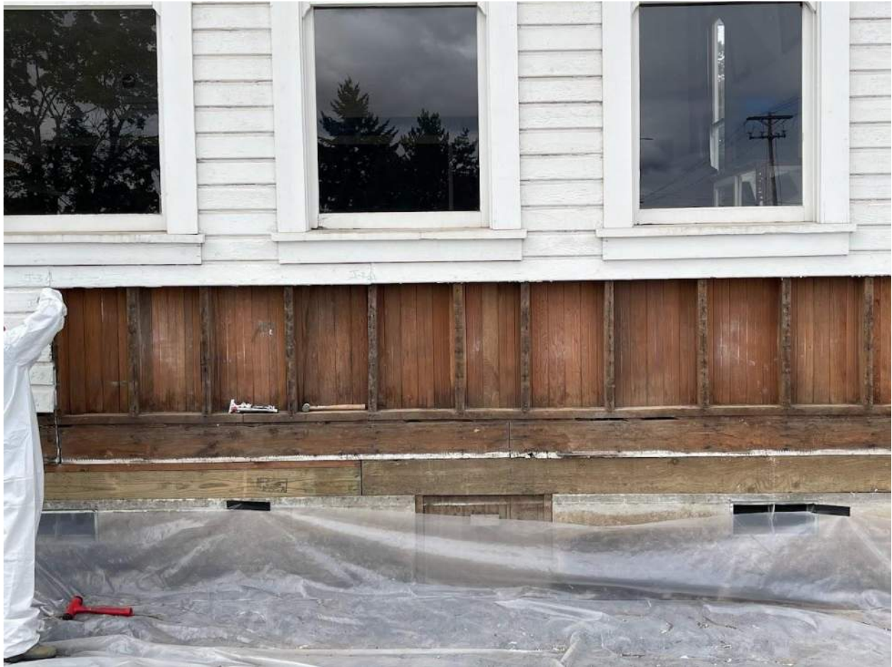
Image 14: Detail of structural system taken during repairs made by Clatsop Community College volunteers. Source: Ryan Prochaska 2023.
