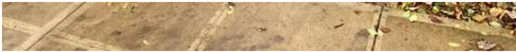
View of the East side with porch under construction. The long side is 10 feet.
