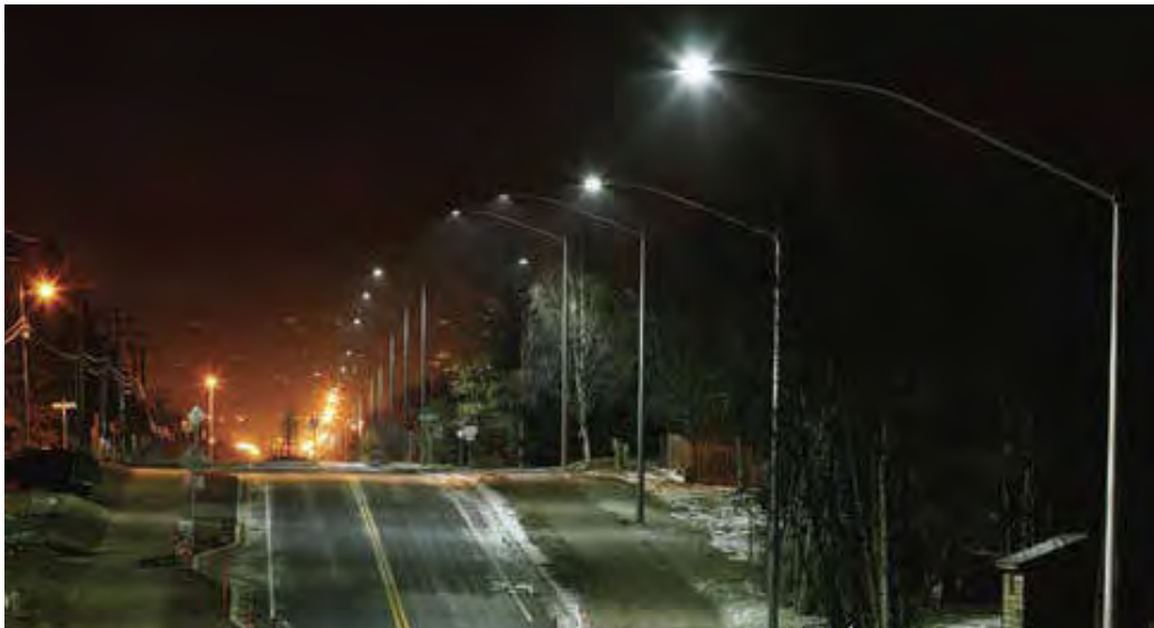
Figure 2: A section of road lit with LEDs, as compared to the HPS lighting in the distance
