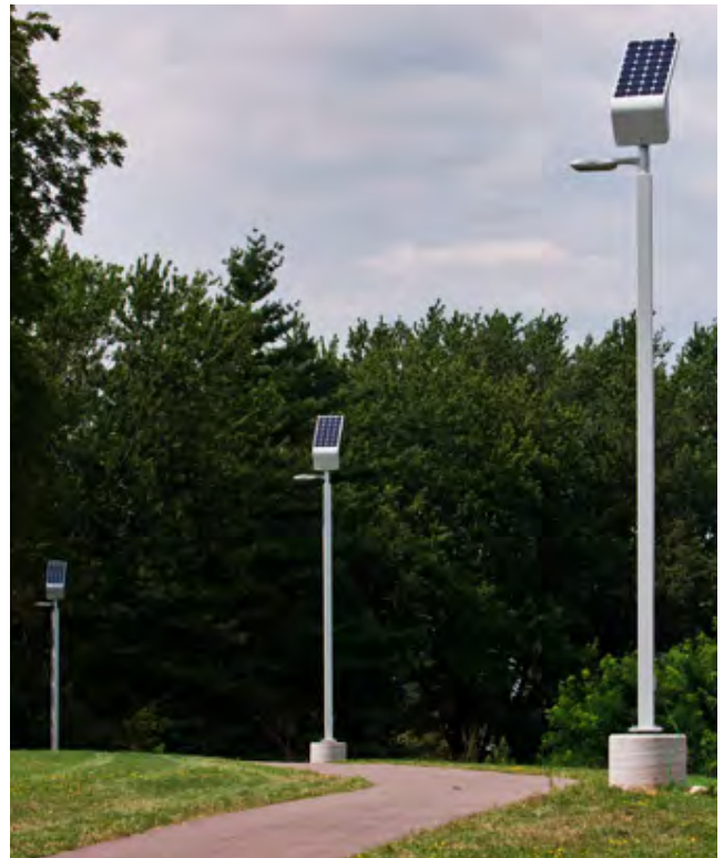
Figure 3: Solar-powered lighting installed in Thut Park in Madison, WI
