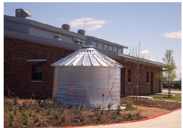
Figure 36: 5,600 gallon rainwater cistern for Denton Fire Station, TX.
