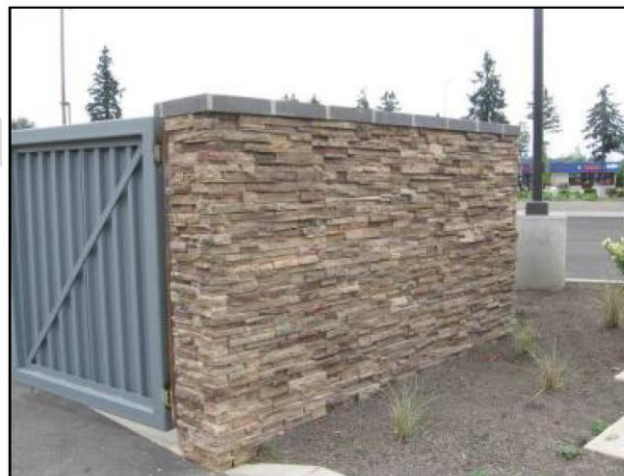
FIGURE 53X-9 GROUND-LEVEL MECHANICAL EQUIPMENT
