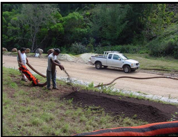
Compost berm being applied in combination with gravel bags as perimeter control.
