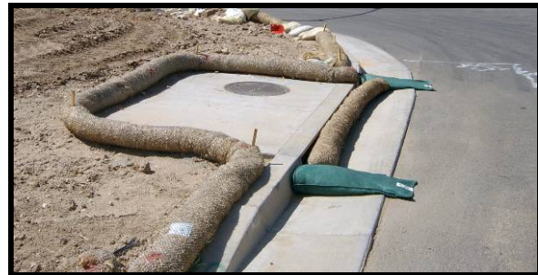
Weighted fiber roll used in combination with heavy duty gravel bags for inlet protection
