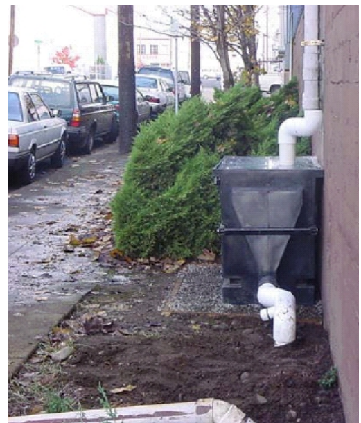
Roof Downspout type filter
